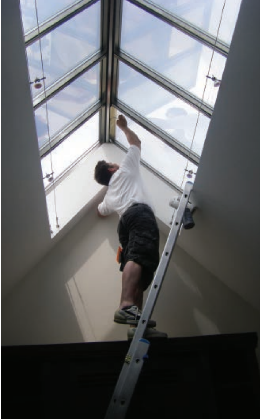
UVR films installed on an atrium (private client)
